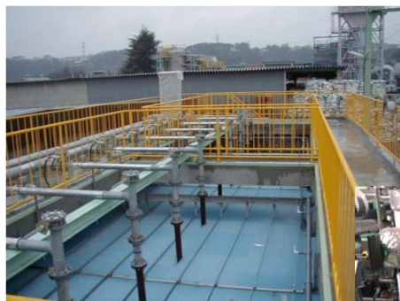
Installation of apparatus for biological treatment and application of its member (carrier)
