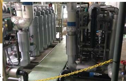
Membrane treatment apparatus installed in the operations
