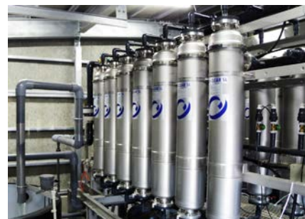
Ultrafiltration facility for removal of chemically formed floc of cadmium.
