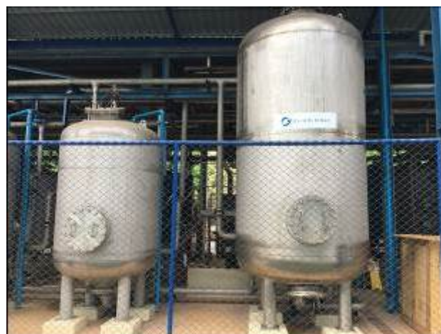
Introduced Water Treatment Facility
