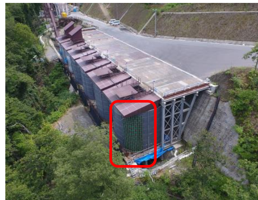
A scene of installation of the cool sheet to the aggregate storage equipment (the cool sheet is installed at the part surrounded by the red frame in the picture.)
