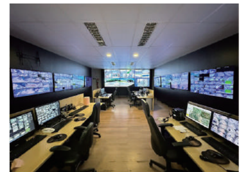
Fire Monitoring Center
